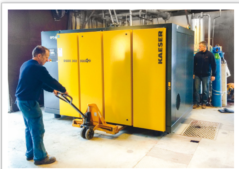
Fig. 1: Arrival of the new helium-gas compressor in the helium liquefaction centre's building at the Institut NÉEL.
